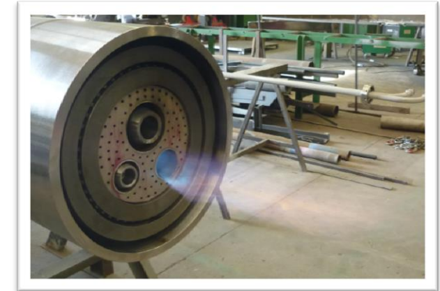
HFO / Methanol – Ignitor trial
