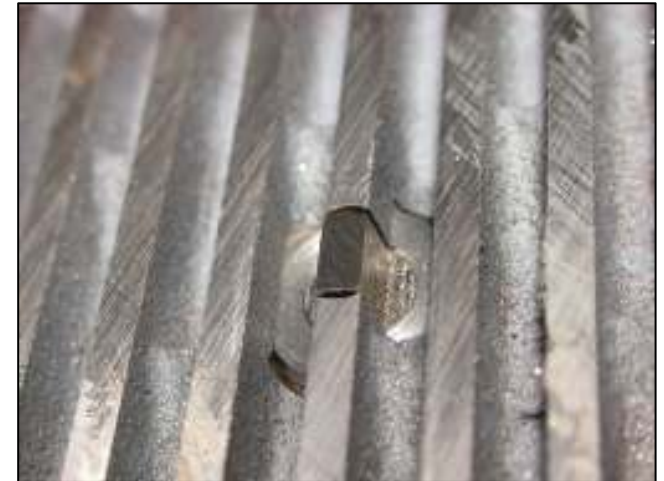
Close-up of RFS4 installed in 45-1B in Port Alberni
