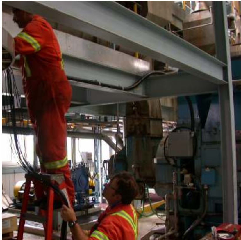
Wire routing to 45-1B refiner at Port Alberni
