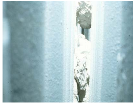
Figure 20. Jammed deposits between tubes in the generating bank
