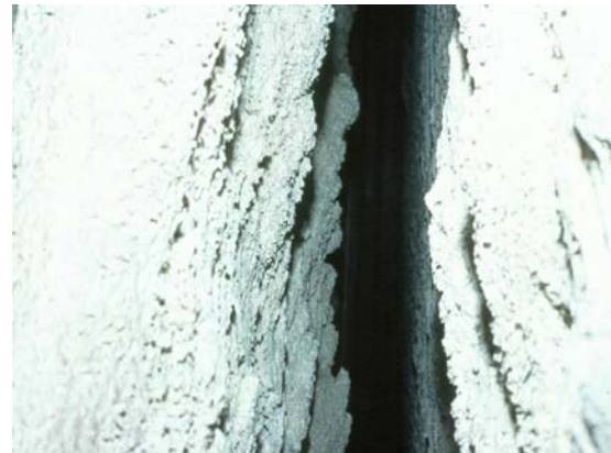
Figure 17. Massive deposit accumulation pattern on superheater platens
