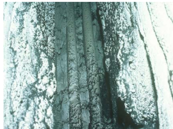
Figure 18. Complete plugging at the generating bank inlet
