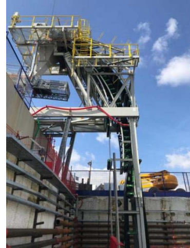
The first of two DSI GPS Sandwich Conveyors elevates 800 t/h of tunnel muck at a 90° angle.
