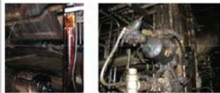
Figure 13 – Leaks have consequences no matter where in the system they occur. Water leak (top) at a pump-pipe fitting, at black-liquor pipe above double suction pump assembly (lower-left), under a pulp slurry pump (lower-right)
